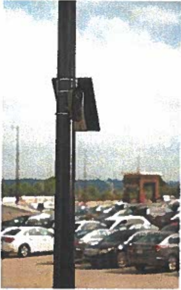
Solar & Existing Pole
